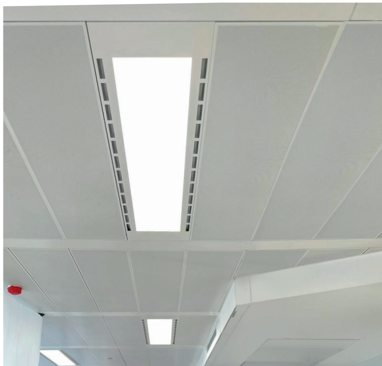
Flatline 1395 x 372mm in Air Handling Frame - SAS330 Ceiling, High Holborn
